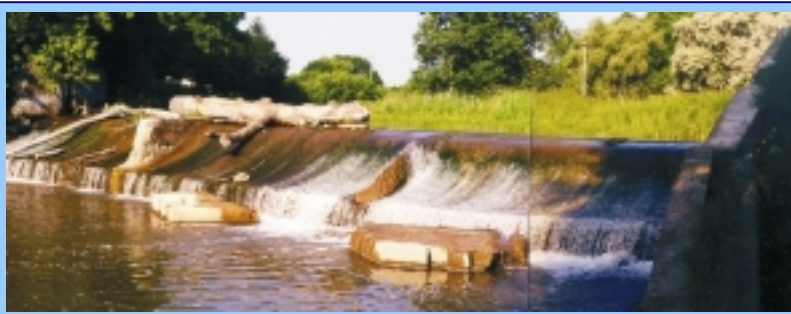
Dams deteriorate over time from the erosive action of water.
